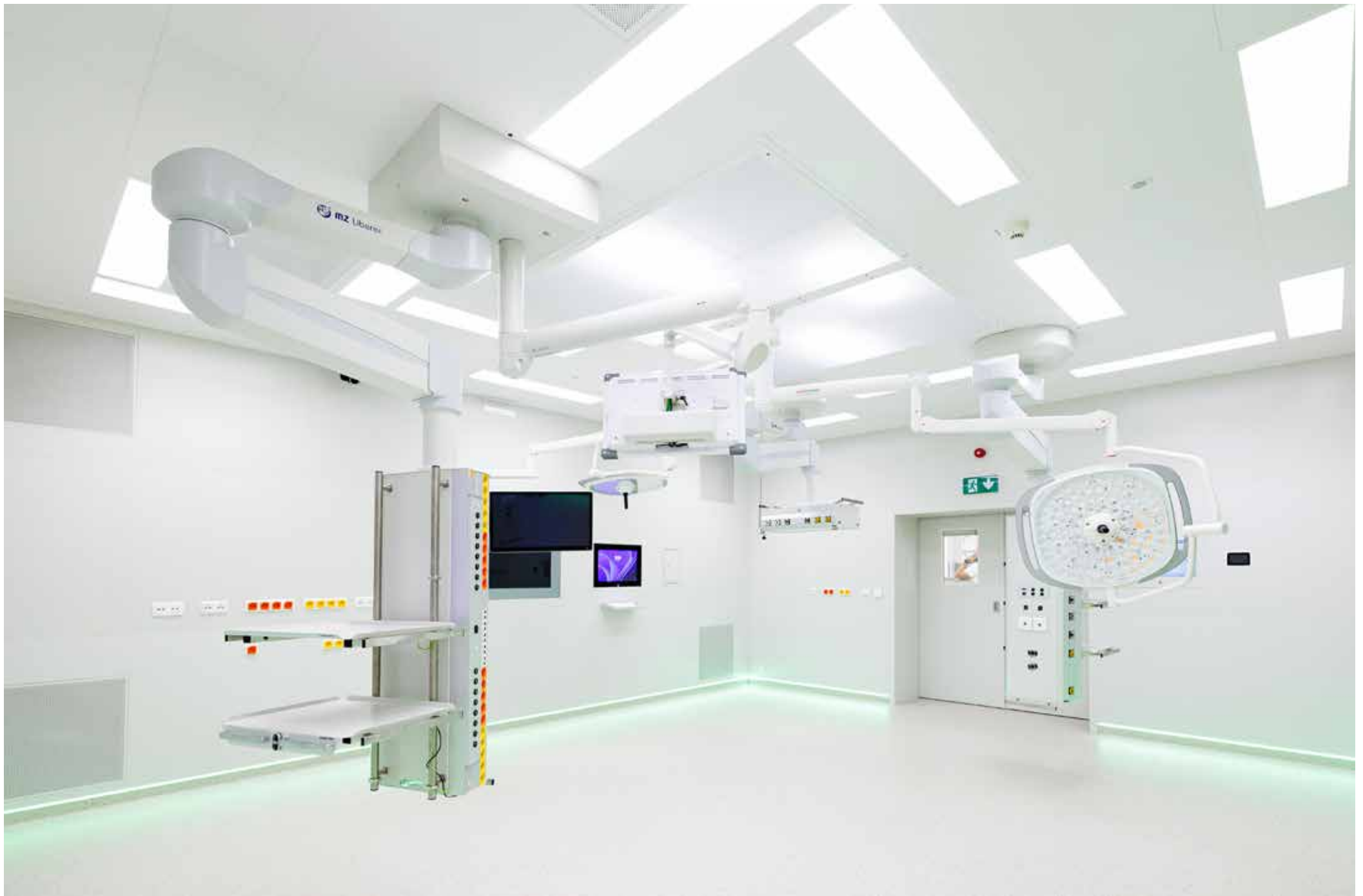
Masaryk Hospital Ústí nad Labem - Operating Rooms | Czech Republic | 2024
